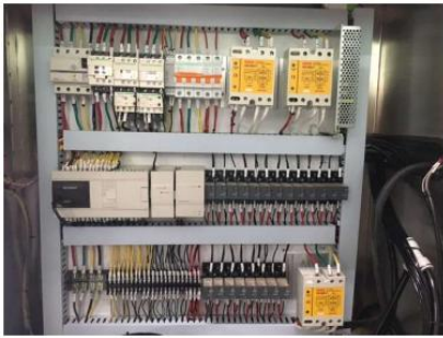
Control Box Mitsubishi,Schneider,CKD,Omron
